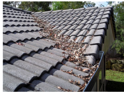
Figure 5. Image of flammable debris on a roof that could ignite from wind-blown embers, reflecting how vegetation near or overhanging structures could increase the likelihood of structure loss.
